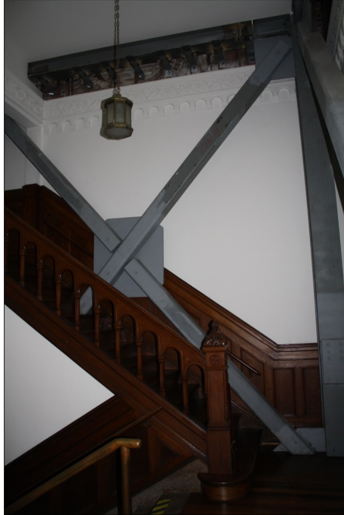
Figure 316. Interior seismic bracing installed in stairwells and hallways off the main nave of subject property.
