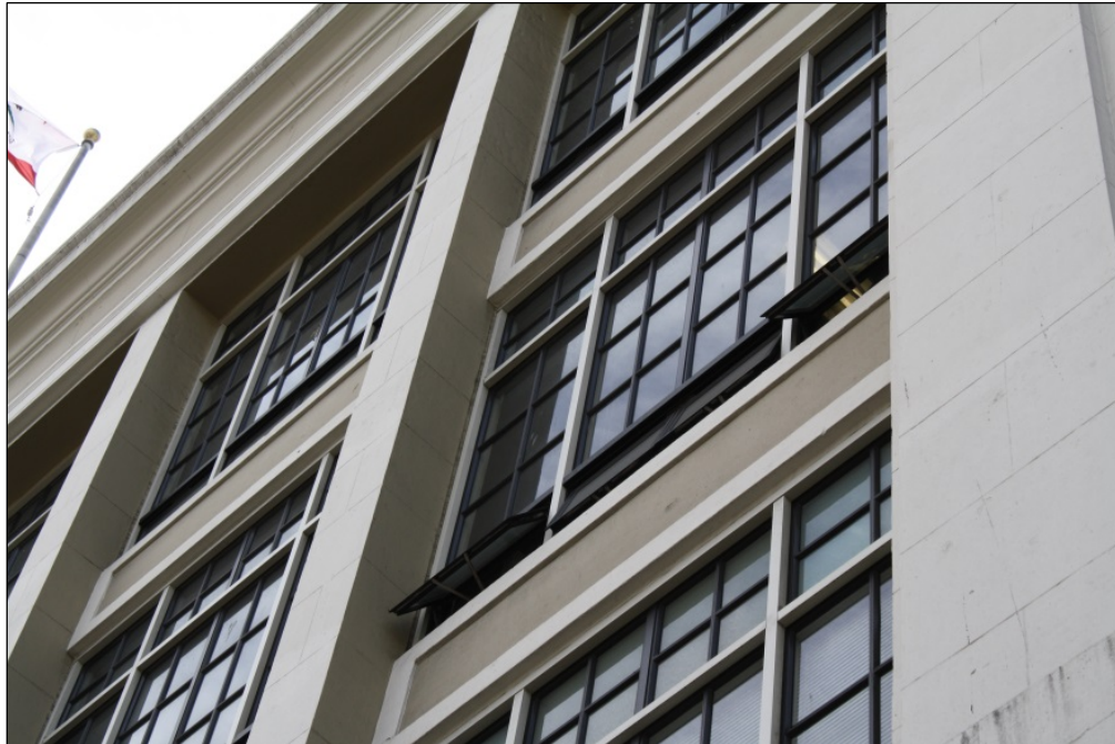
Figure 285. 1849 Van Ness Avenue, close up of the windows on the primary elevation.
